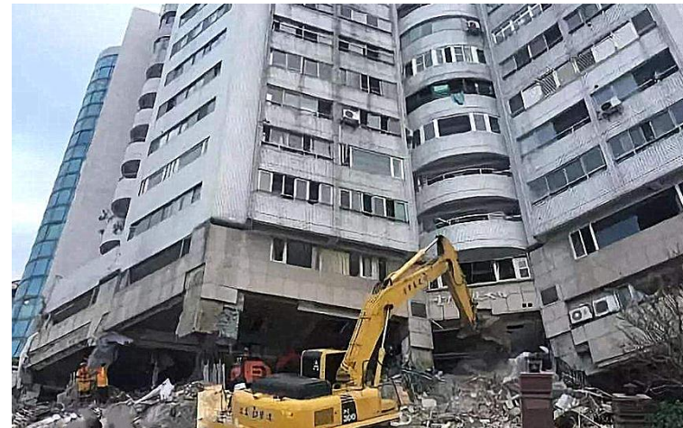
Inaccurately designed building structure
